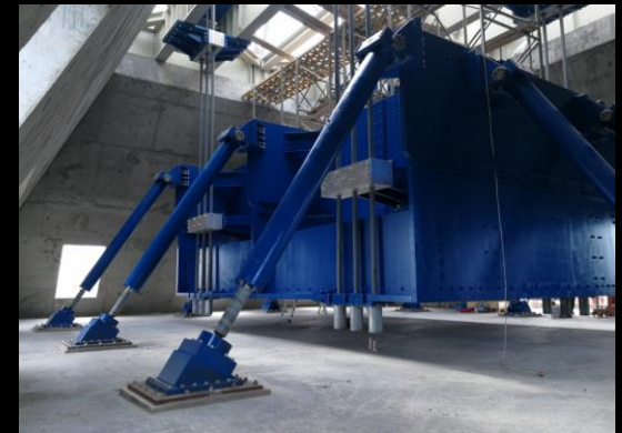
Tuned Mass Damper, Baku Tower, Maurer
